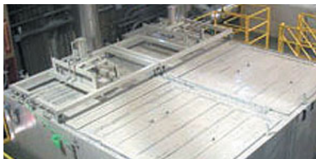
Techni-Cast’s combined-heat-and-power system uses waste-heat from electrical generation to pre-heat metal before melting, thus reducing the overall energy requirements of foundry operations.
